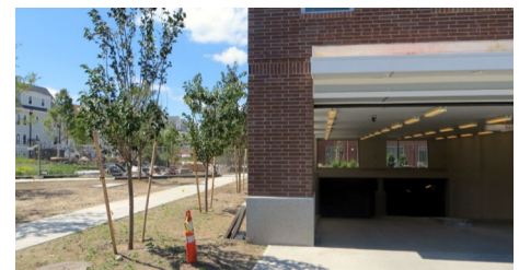
Only the garage entrance reveals that the courtyard is located on a roof surface.
