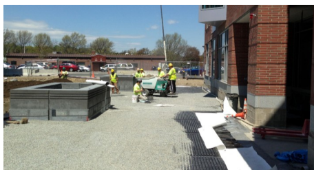
The drainage element Stabilodrain® SD 30 has been applied on the entire roof surface and completely filled with stone chippings.
