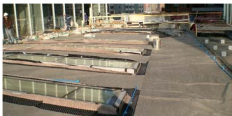
The irrigation pipes were installed above the filter sheet, the entire surface beneath is covered with Floradrain® elements.
