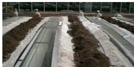
The growing media and the gravel (for the edges) are distributed evenly all over the roof surface.
