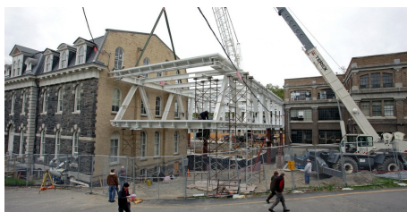
The new building is based on a steel-glass-structure and its main purpose is to connect the two buildings in which accommodate the architecture department.
