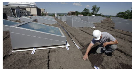
After the laying of the drainage elements on the entire roof surface the growing media providing the base for the plants has been applied.
