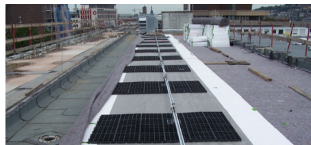
The ZinCo ballast held fall protection system was installed on the upper green roof area.
