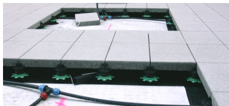
Under the elevated concrete slabs was enough space for the irrigation pipes.
