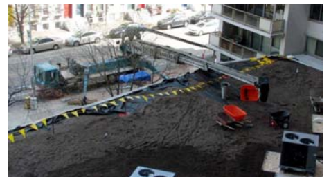
The substrate was transported to the roof via a telescopic conveyor belt (Telebelt).
