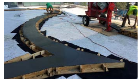
Floradrain® FD 40-E was used as a permanent formwork for the curb and seatwalls.
