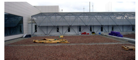
The roof area just after the application of substrate with Big Bags.
