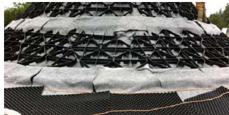
The Floradrain® elements adjacent to the sloped roof area where Georaster® was applied.
