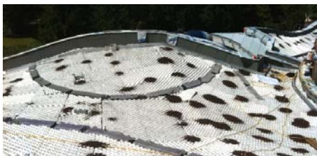
The roof of the visitor center shortly after the installation of the Floraset® FS 75 elements.
