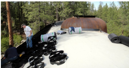
In the steeper areas the Georaster®-elements have been placed on the Water Retention Mat WSM 150, starting from below.
