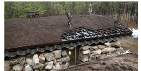
In the next step the drainage elements were completely filled with the growing media.
