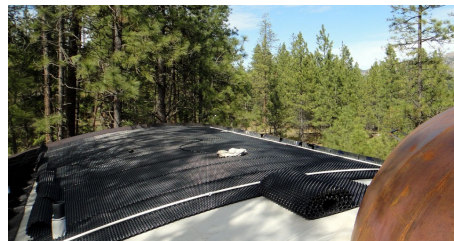
In the flatter areas above the Georaster®-elements Floradrain® FD 40-R have been installed.
